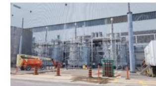
A look at new transformers installed at Darlington Nuclear's Unit 3 in July 2021.
