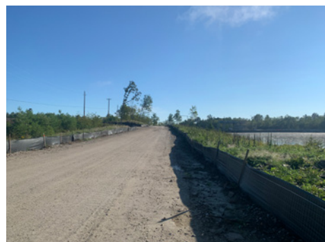
(Left) A silk fence helps keep out any wildlife from the area, including species at risk, while protecting them from entering into the busy construction zone.
