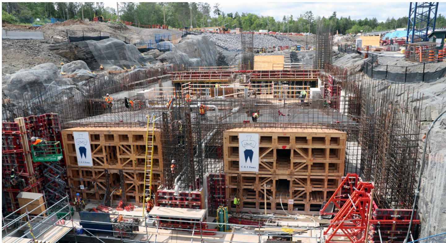
(Above) A view looking upstream at the new powerhouse draft tubes under construction.
