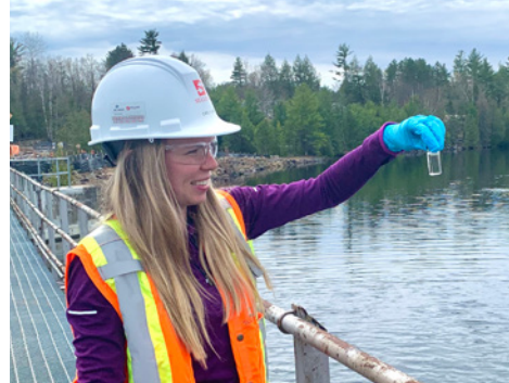
(Left) Carly Lance, a Junior Health, Safety and Environment Assistant with contractor M. Sullivan and Son, examines a water sample at OPG's Calabogie Redevelopment project site.
