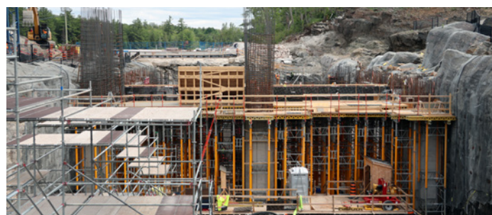
(Above) A view looking downstream at the new generating station under construction. Most notable are the many vertical shoring posts, ready to support the intake soffit and upper slab formwork. Water will eventually flow into the intake structure and through the generating units to produce electricity.
