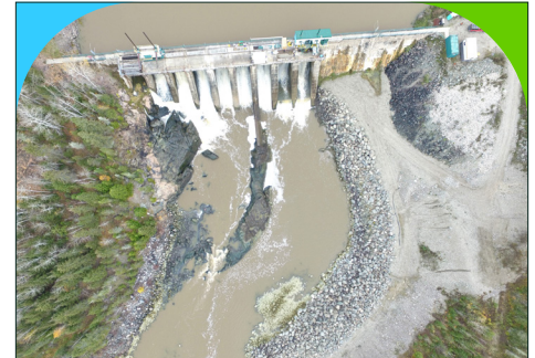
The Frederick House Lake Dam Rehabilitation Project is 39% complete, with work continuing into 2025.
