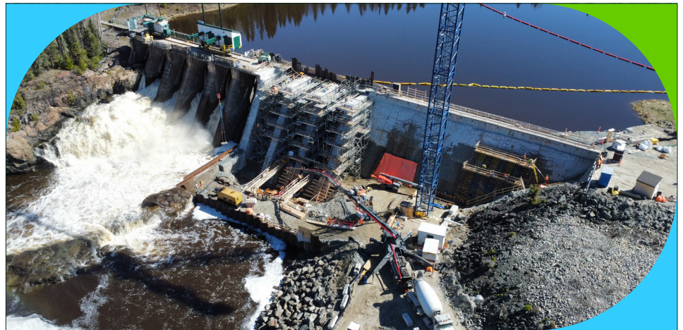
Construction at Frederick House Lake Dam is well underway, with several construction milestones completed for Phase 1.
